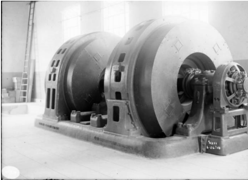
Figure 18: Interior Capistrano Substation, frequency changers, June 26, 1918.
