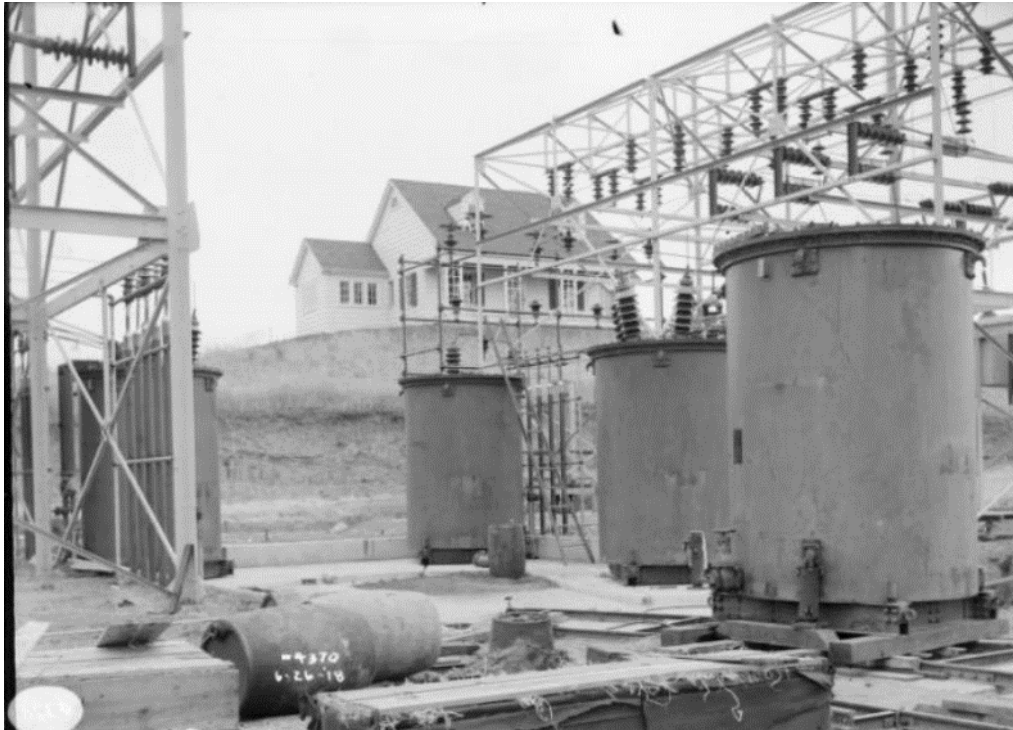
Figure 14: Racks and transformers, June 26, 1918.
