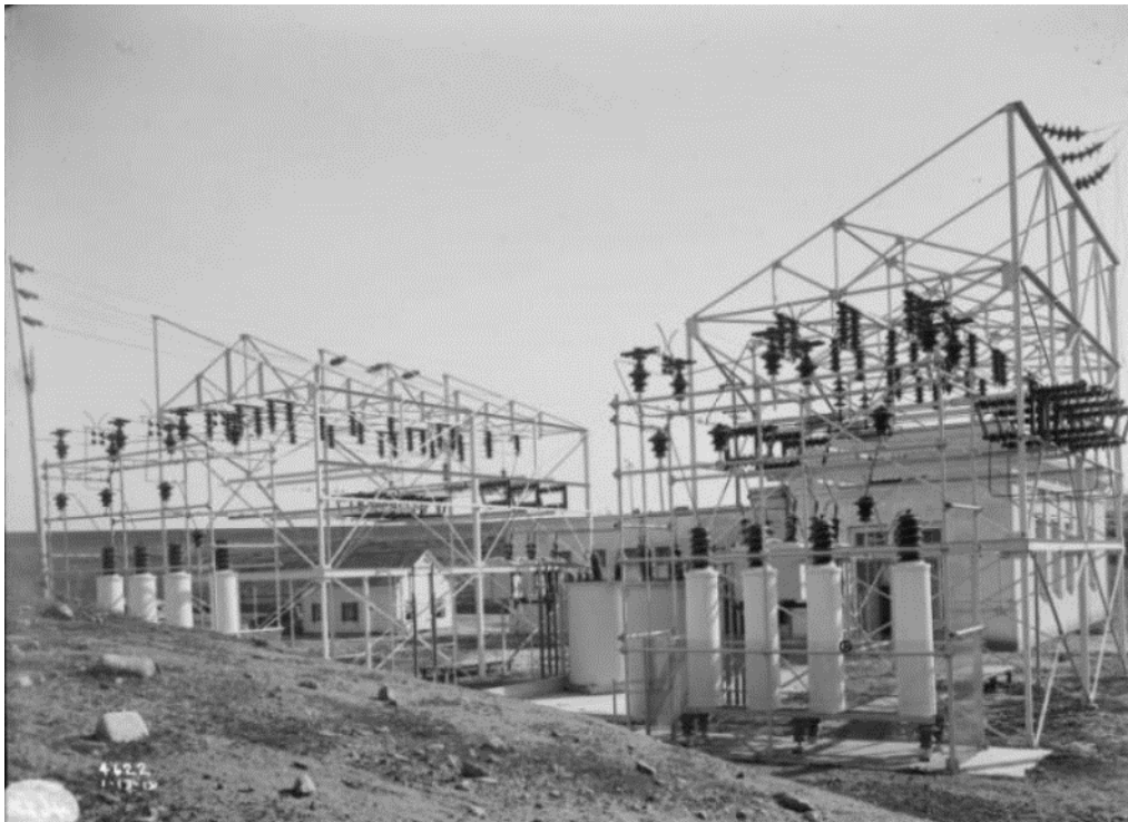
Figure 15: Arresters, racks, and transformers, January 13, 1919.
