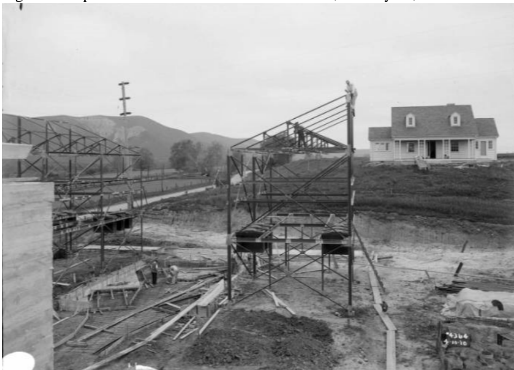
Figure 7: Capistrano Substation showing exterior equipment racks under construction with operator's cottage upper right, April 10, 1918.
