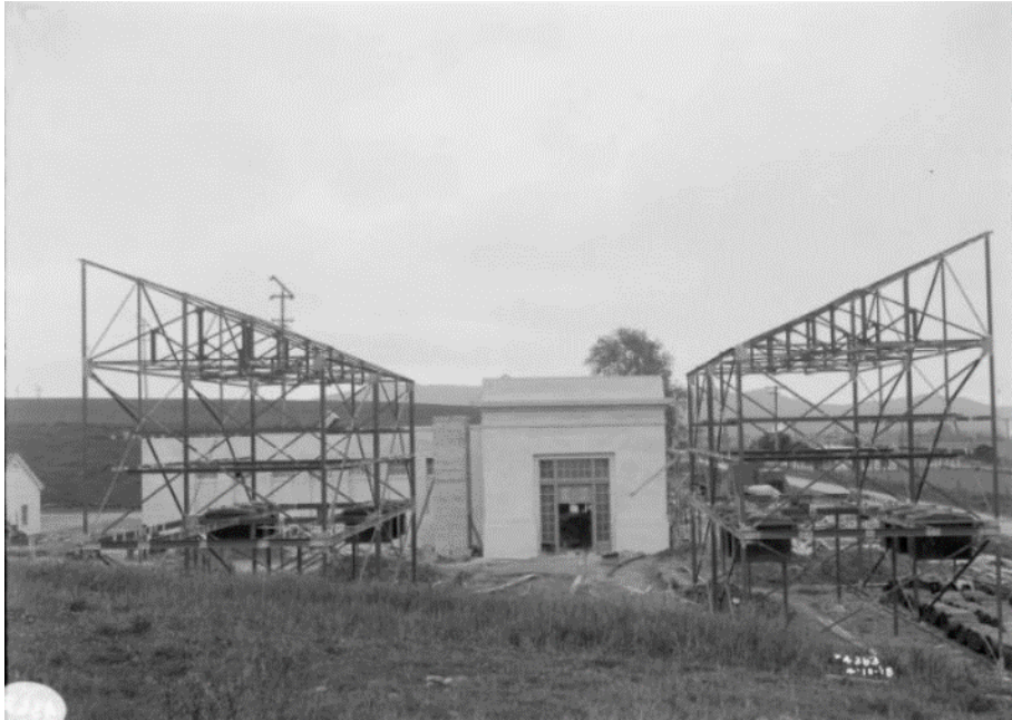
Figure 8: Capistrano Substation showing exterior equipment racks, April 10, 1918.
